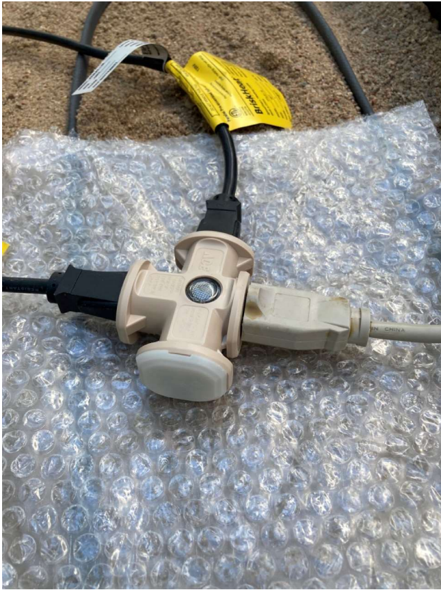
Fig 9. Y-connector with control cable coming from right, two heat cables
